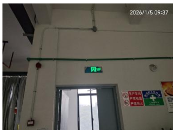
Fire alarm, Exit sign and emergency light.jpg
